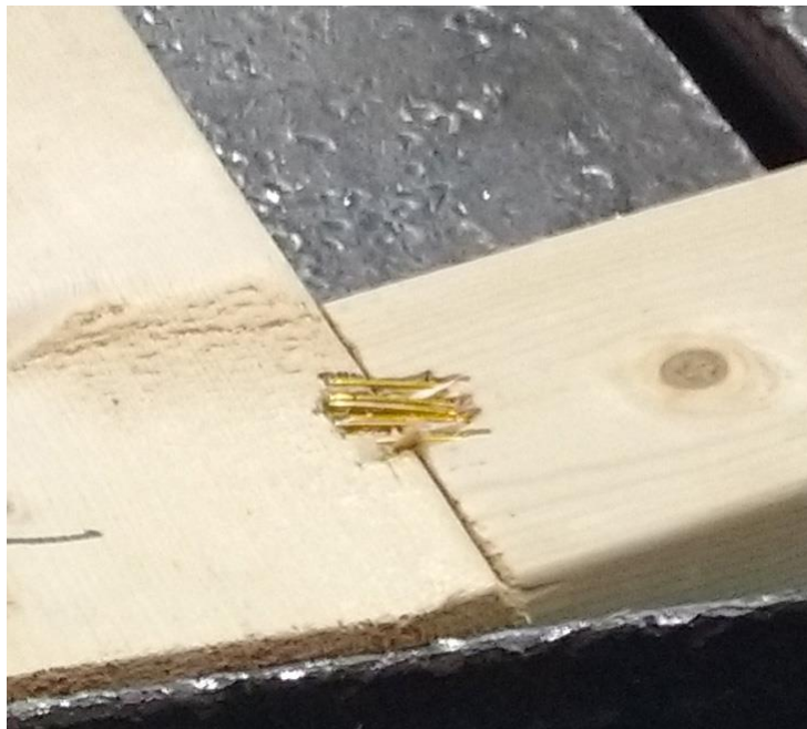
Too many staples at this joint
