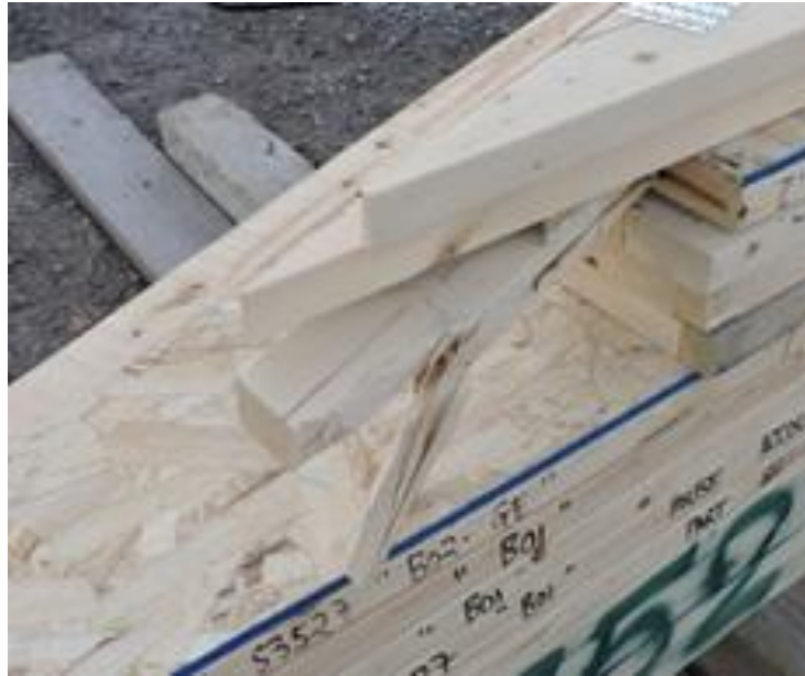
Damaged trusses prior to delivery
