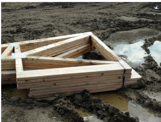
Trusses moved by the builder into the mud
