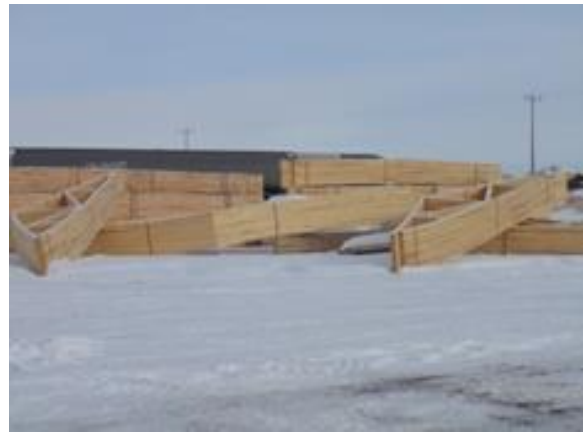
Trusses not stored properly
