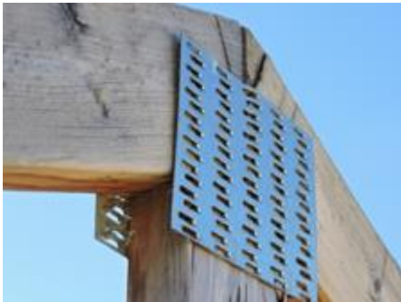
Trusses left exposed to the weather
