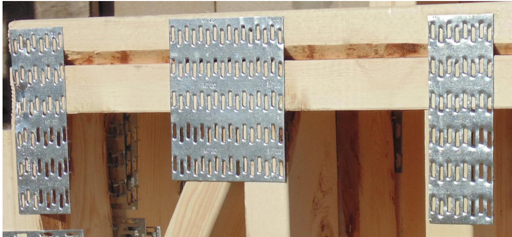
Wane in top chord resulting in ineffective teeth
