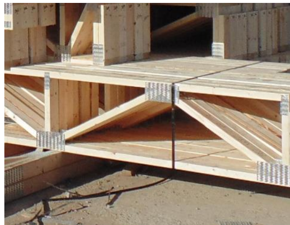
Improper banding in mid panel
