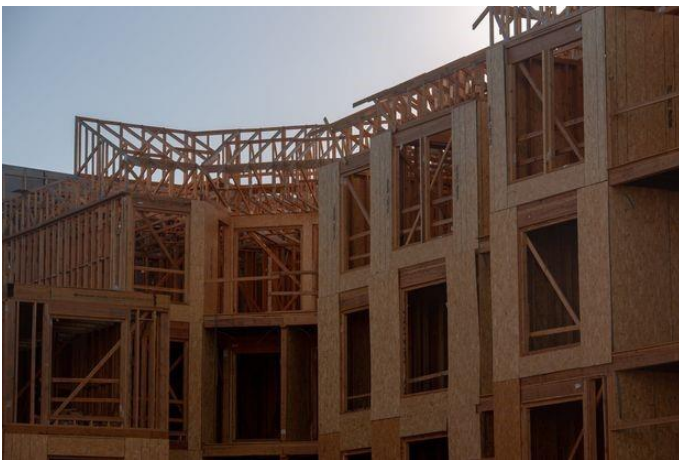
Katerra's Legacy at Livermore construction site, pictured on June 26, in downtown Livermore, Calif. The site now sits unfinished after the company declared bankruptcy in June.
